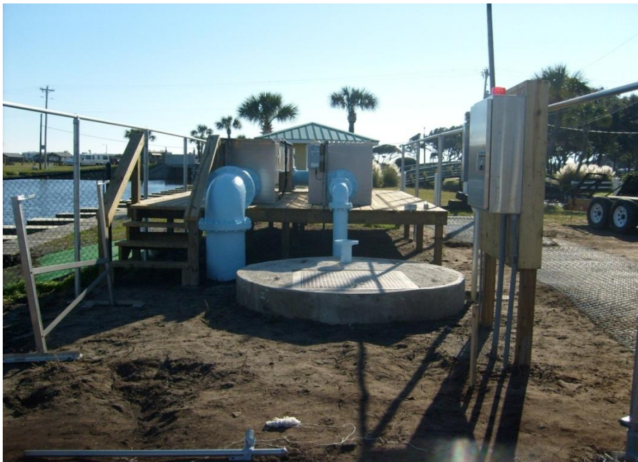
Figure 5 – End View of UV unit showing intake and outlet piping, and pump station
