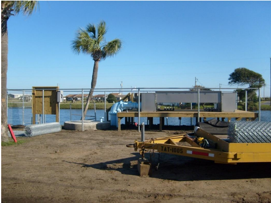
Figure 4 – Side View of UV Units prior to fence enclosure
